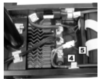
Plug at controller
